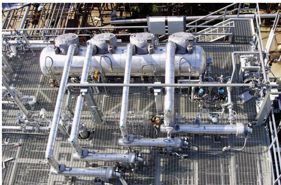
FIG. 1. A sulfur-recovery unit in the field.
